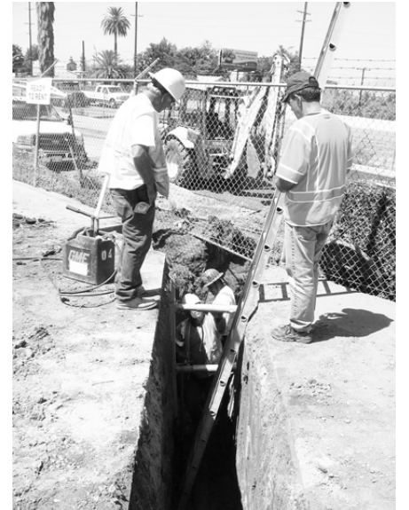
Workers are shown connecting the RSC rental yard to the new sewer line on East La Cadena Drive.
