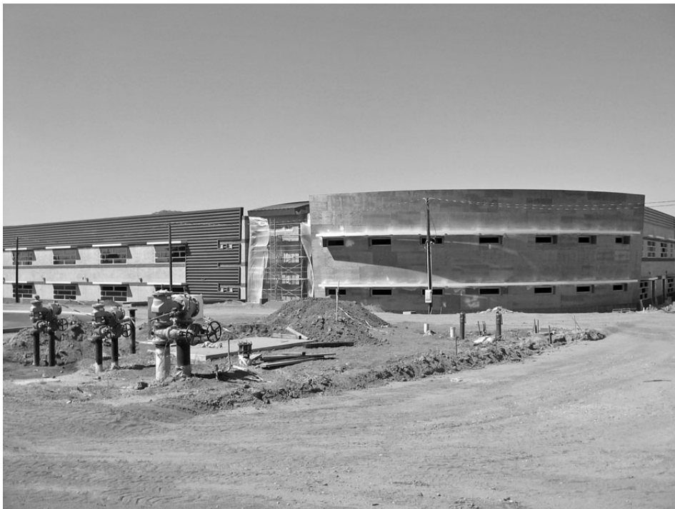
The $143 million dollar High School is set to open in 2012 on the north side of Main St. which is the boundary between Grand Terrace and Highgrove.
