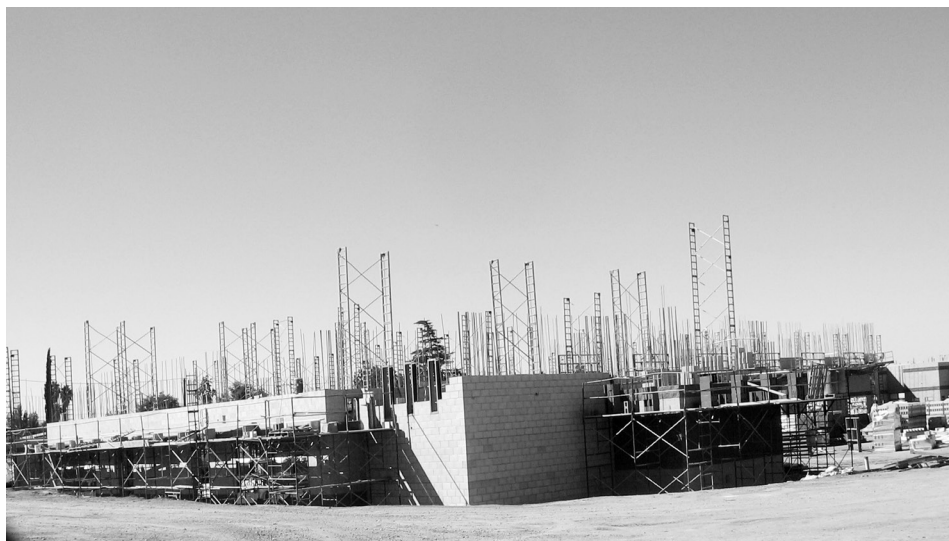
Some of the buildings are about half way of reaching their height.
