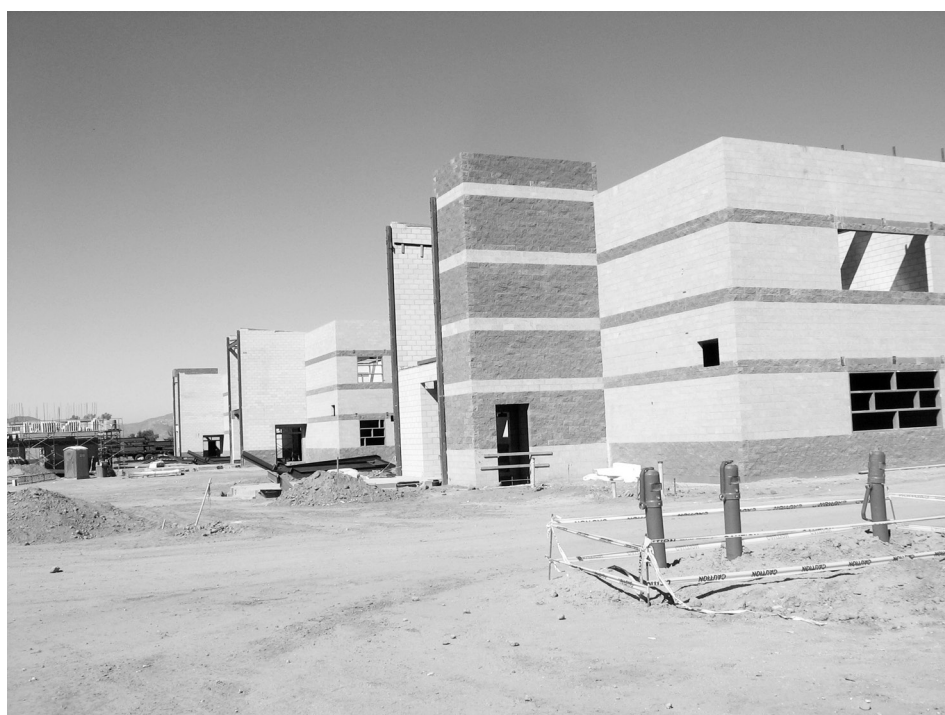
Other buildings are almost completed but there is still a lot to do!
