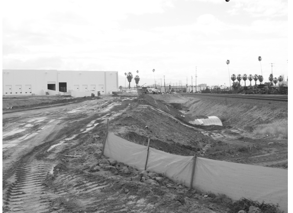
The purpose of the pipe is for a future trail in this area to provide the safe passage of animals and people who want to use the trail system that is being planned. However, at this time the huge pipe does not go under the railroad track. The pipe ends between the new dirt landfill road and the BNSF RR tracks main lines.
