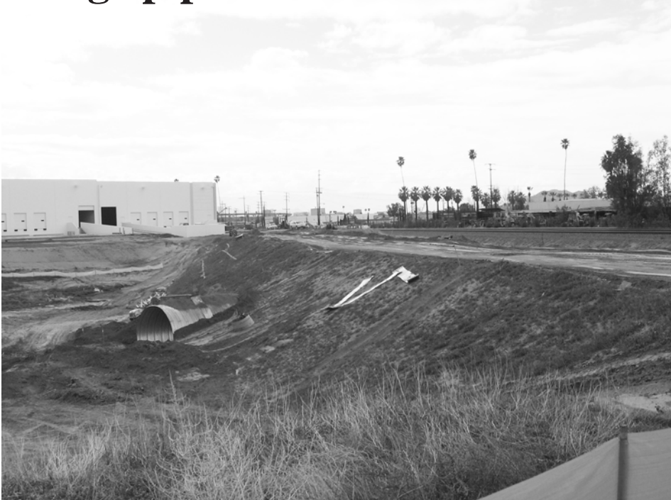
A 12 foot diameter pipe has been installed under the new dirt roadway that was created across the arroyo during the construction of the new large warehouses on the north side of Citrus Street. This view is on the east side of the new road.
