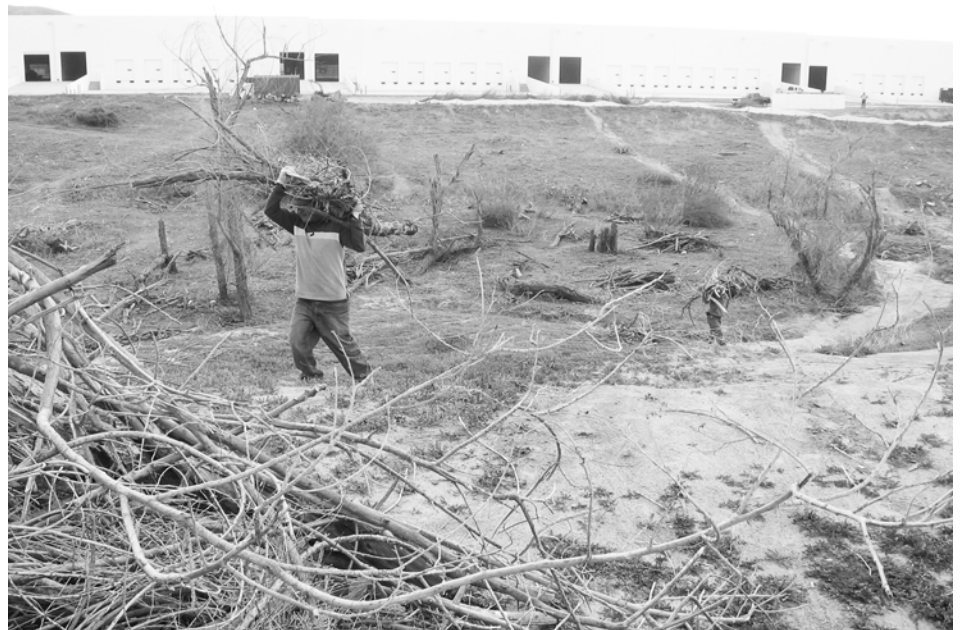
Another project in the arroyo north of the new warehouses on Citrus St. is the removal of dead vegetation in the Spring Brook Wash arroyo. This is part of Riverside Commercial Investors efforts to clean and replant the arroyo with new vegetation that is native to the area. This view is looking south across the arroyo to the back of the new warehouses on Citrus Street. Directly behind the photographer is the 19 acre parcel of vacant land that has been mentioned so many times in reference to the land that is needed for the curved track that will connect the Perris Valley Line RR to the BNSF RR and where a Highgrove Metrolink station stop is wanted and needed. The dirt roadway across the arroyo is scheduled to be paved soon, when the parking lot for the new warehouses are paved.
