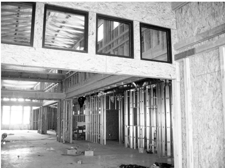
The inside will be beautiful and have about 7 times more room than the old one.
