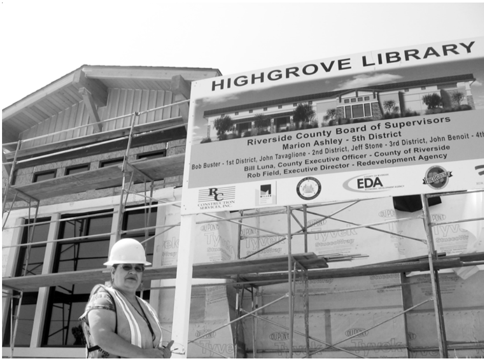
Louise Gutierrez, Highgrove librarian, and I were given a tour of the new 7,000 sq. ft. library that is under construction at Center St. and Michigan Avenue.
