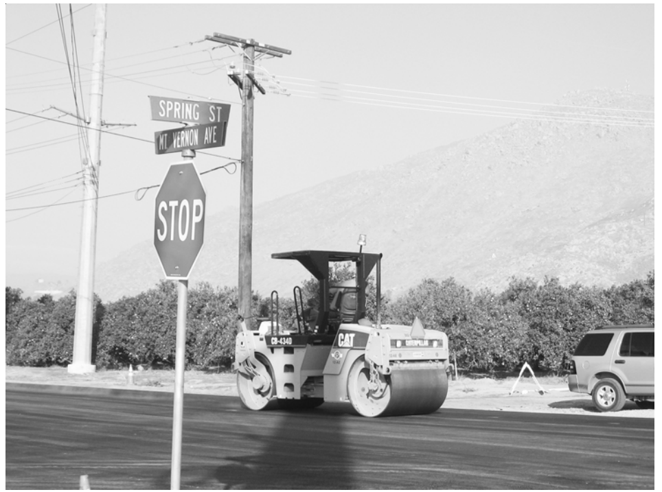
The new pavement was compacted by this machine and now its nice and smooth
