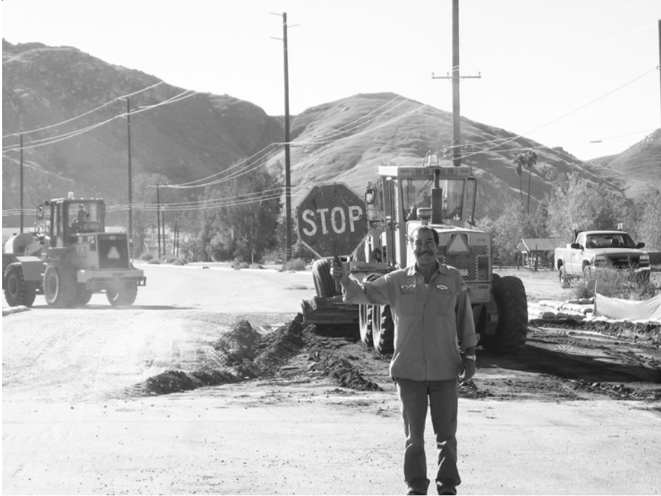
Hugo Munoz, a crew member of the Riverside County Transportation Dept. directed traffic on Dec. 1, 2008 during the repaving of the intersection.
