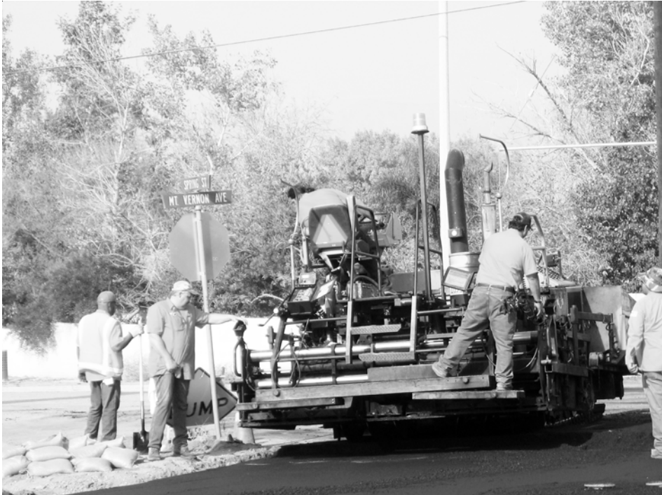
The crew above is shown using the asphalt paving machine at the corner of Mt. Vernon and Spring Street. There are large pipes under this intersection that were placed there as part of the flood control portion of the Spring Mountain Ranch grading and portions over the pipe had settled making the pavement uneven. The potholes were filled several weeks ago and now the new asphalt has made the intersection nice and smooth and will enable traffic to get from Mt. Vernon Ave. to Palmyrita Avenue.
