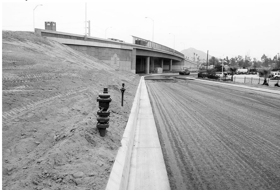
The Iowa overpass is shown here on the east side looking toward Highgrove during the paving on top of Iowa Ave. and the streets below the overpass.
