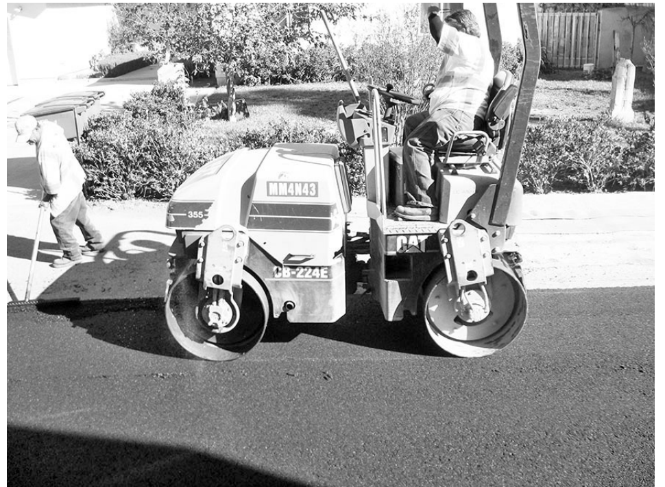
The final portion of the paving is when the roller makes everything smooth.
