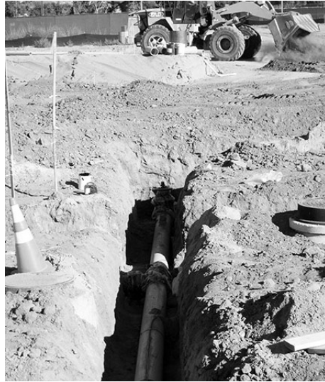
The underground sewer lines, water lines and other lines are already in.
