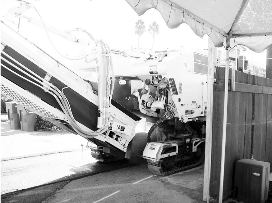
The old pavement is chipped up and loaded it into a truck and hauled away.
