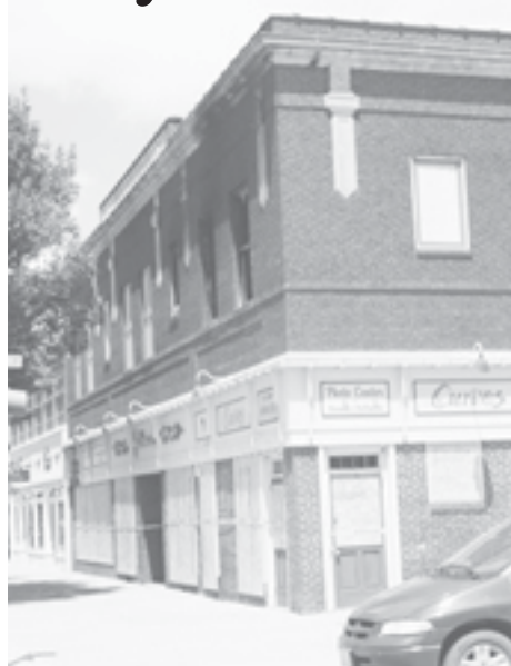
After the fire, fortunately the brick walls are still standing.
