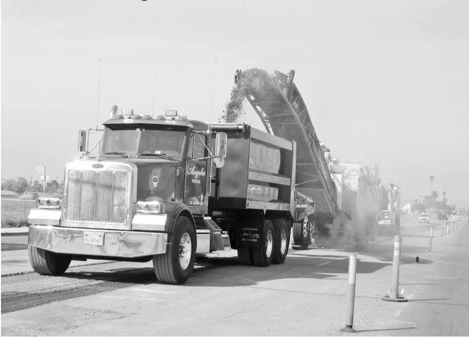
The machine in the rear chips the asphalt onto a conveyor and into the truck so the patched surface will be the same level as the roadway.
