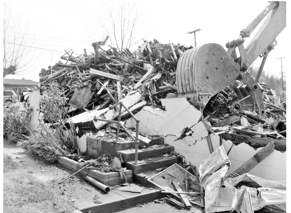
A few minutes later the house was eaten away by this giant biting machine. The center of the picture shows the steps and hand rail to the north side of the house. This property is now vacant land except for the rock planter around the boundary along Main St. and Michigan Avenue.
