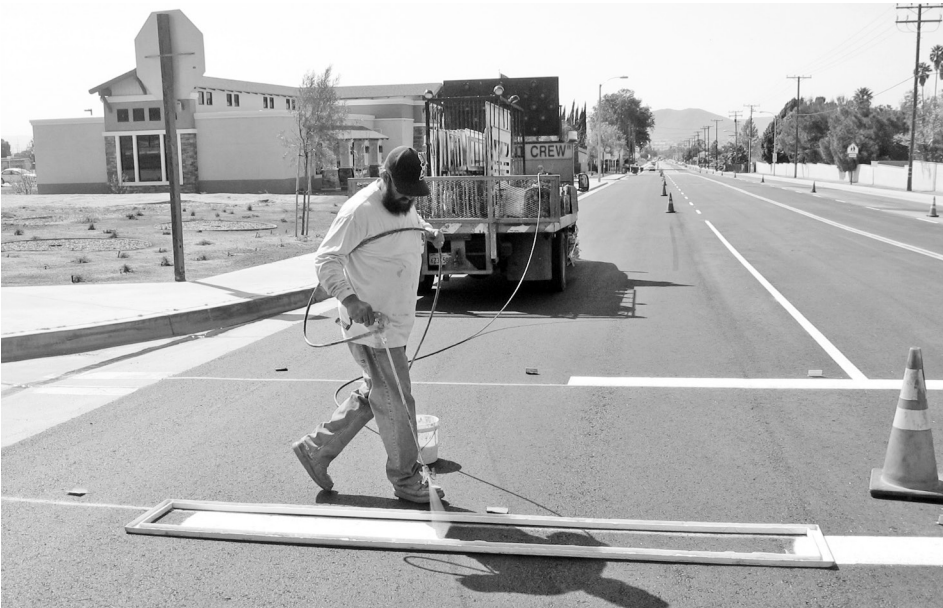
After the asphalt was chipped away, portions of Center St. were repaved and new traffic lanes and crosswalks were repainted on Center Street.
